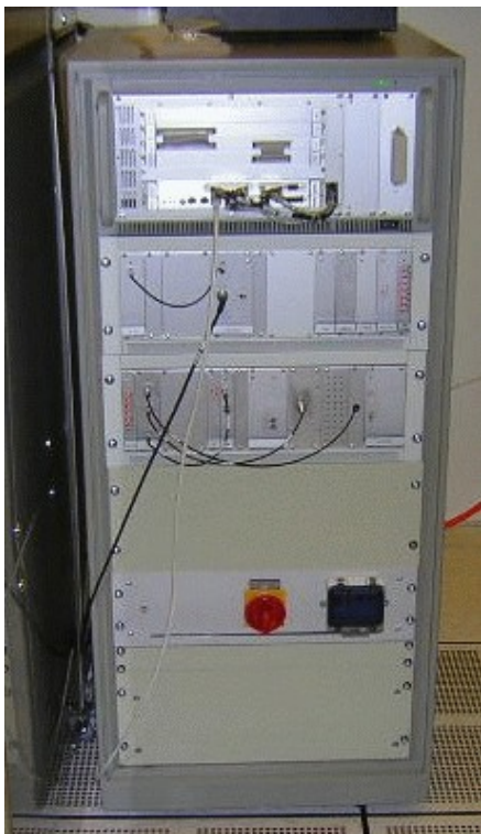
Figure 1-2: Exposure Control Computer rack
